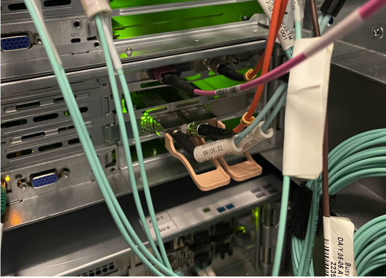
Figure 7.4: Photograph of the FELIX card used for the Tile Demonstrator readout. Visible connections include the MTP fiber (purple) for data transmission and clock distribution, and the ST fiber (orange) receiving the clock signal from the Tile LBA ALTI system.
