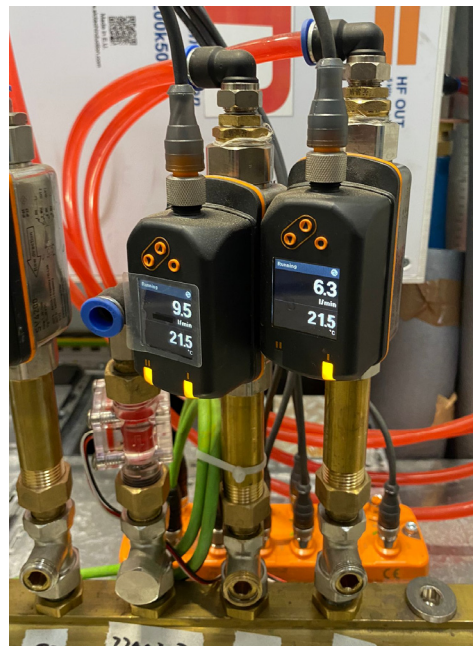
Figure 8. Pressure, flow, and temperature sensors.
