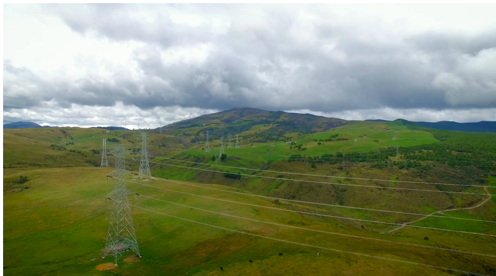
Figure A.19: Substation and transmission lines.
