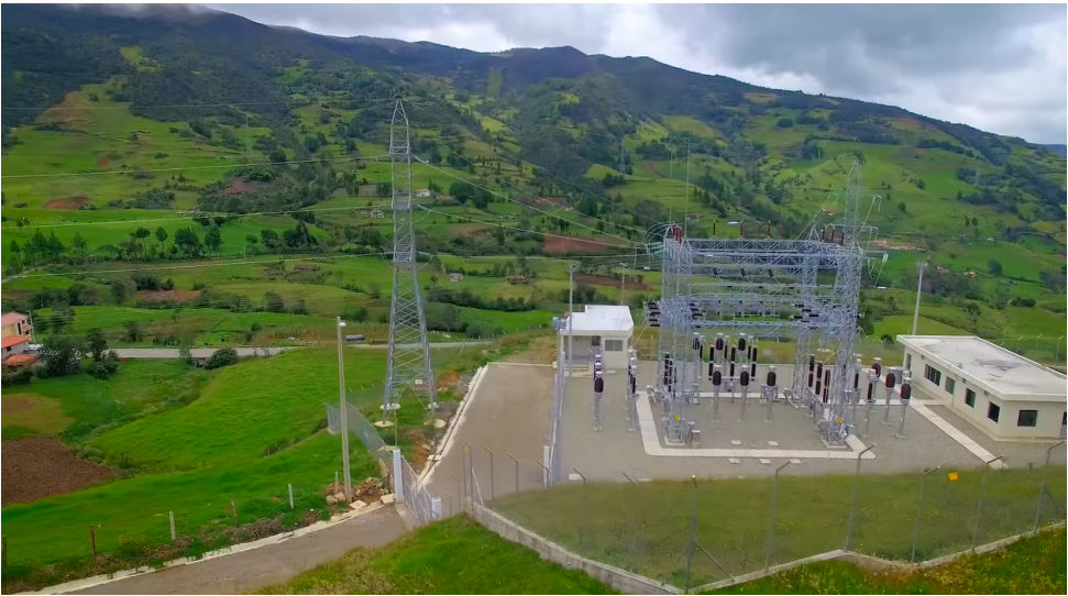
Figure A.18: Substation and transmission lines.
